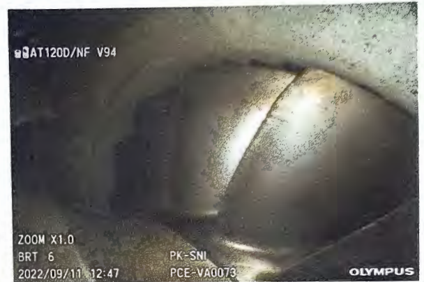
Photo of First Stage Compressor 4 th Quadrant
