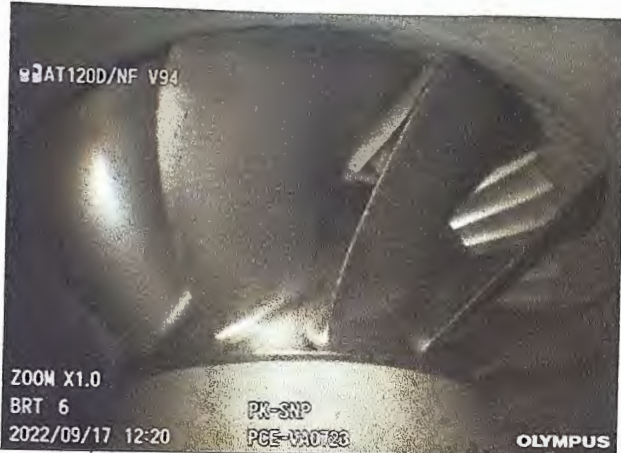
Photo of First Stage Compressor 3 rd Quadrant
