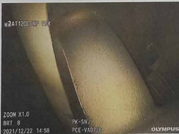
Photo of CT Stator 3 rd Quadrant
