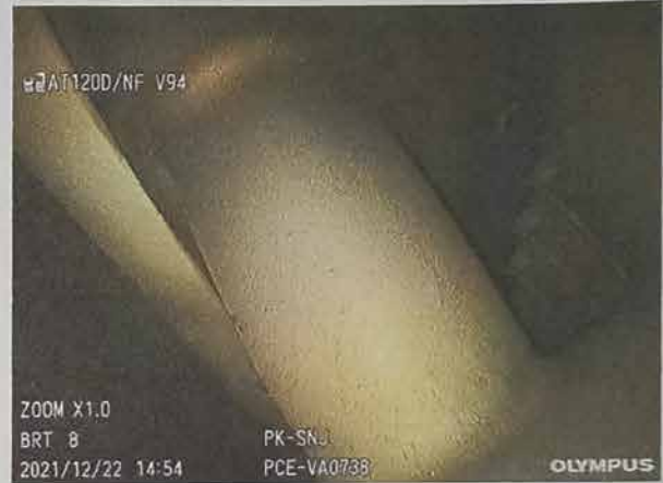
Photo of CT Stator 2 nd Quadrant
