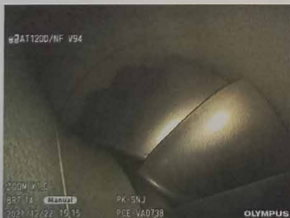
Photo of First Stage Compressor 1 st Quadrant
