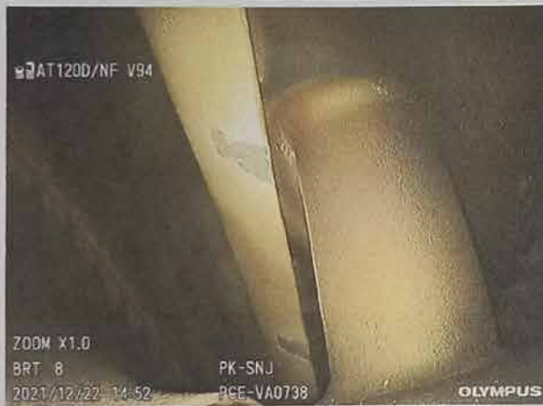
Photo of CT Stator 1 st Quadrant
