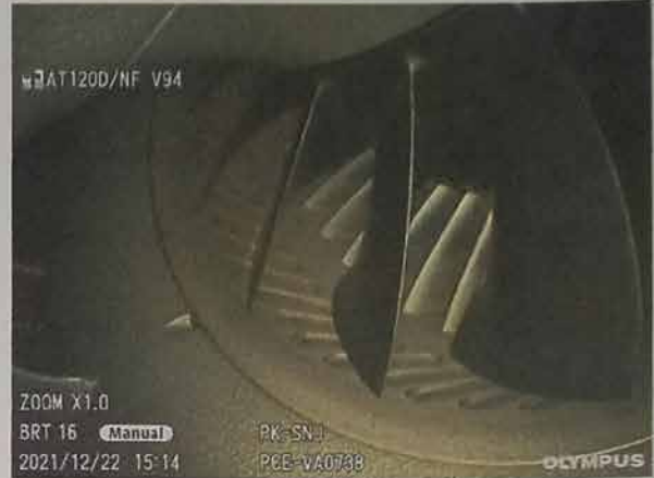
Photo of First Stage Compressor 4 th Quadrant
