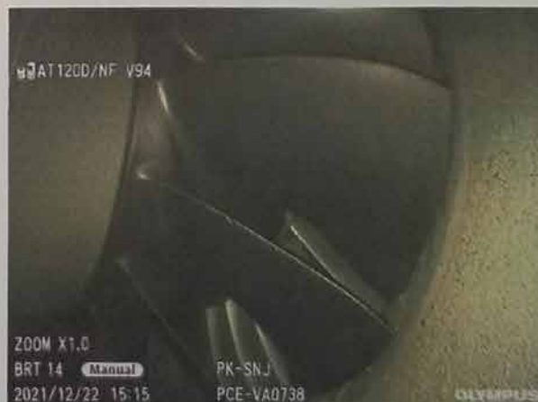
Photo of First Stage Compressor 2 nd Quadrant
