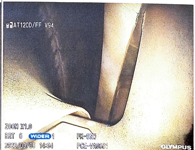
Photo of CT Stator 2 nd Quadrant
