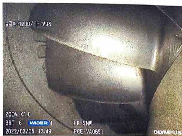
Photo of First Stage Compressor 2 nd Quadrant
