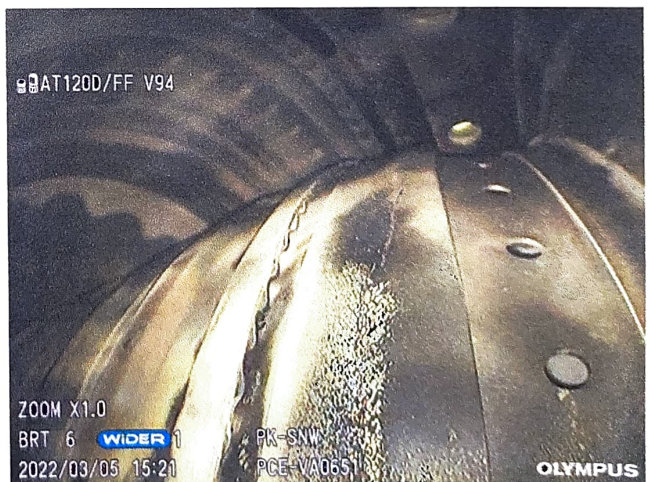
Photo of Combustion Chamber 2 nd Quadrant
