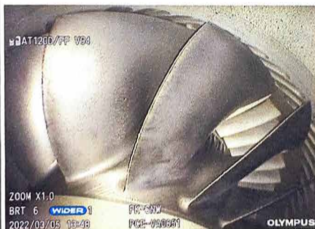
Photo of First Stage Compressor 1 st Quadrant
