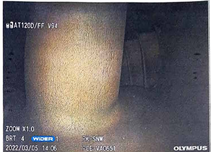
Photo of CT Stator 4 th Quadrant
