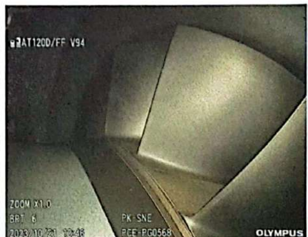
Photo of First Stage Compressor 2 nd Quadrant
