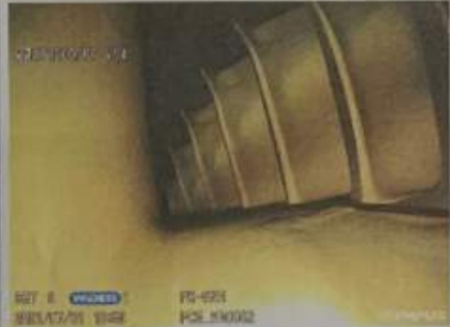
Photo of Leading Edge CT-Blades 4 th Quadrant
