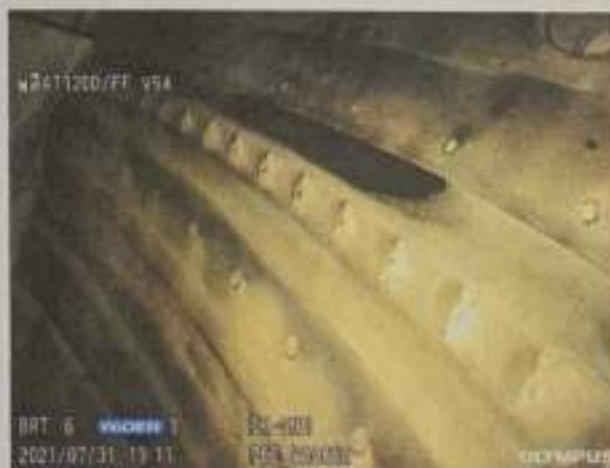
Photo of Combustion Chamber 2 nd Quadrant
