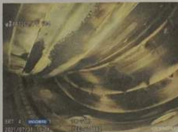
Photo of Combustion Chamber 4 th Quadrant
