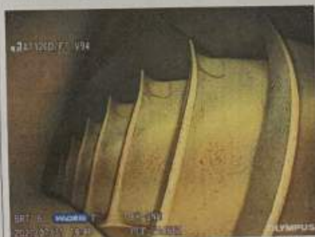
Photo of Leading Edge CT-Blades 1 st Quadrant
