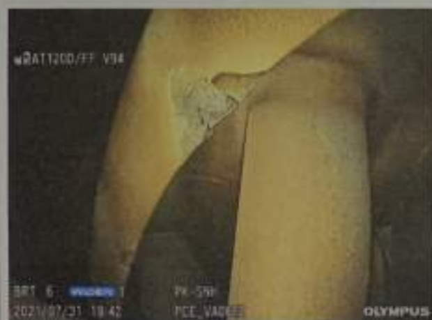
Photo of CT Stator 1 st Quadrant
