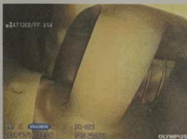
Photo of CT Stator 2 nd Quadrant
