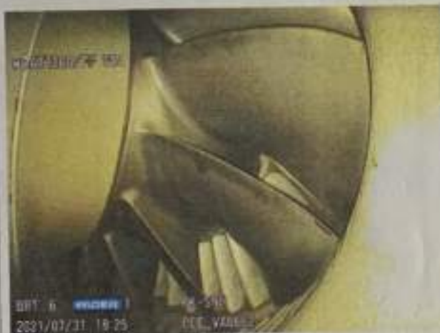
Photo of First Stage Compressor 1 st Quadrant
