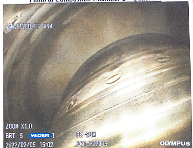
Photo of Combustion Chamber 2 nd Quadrant
