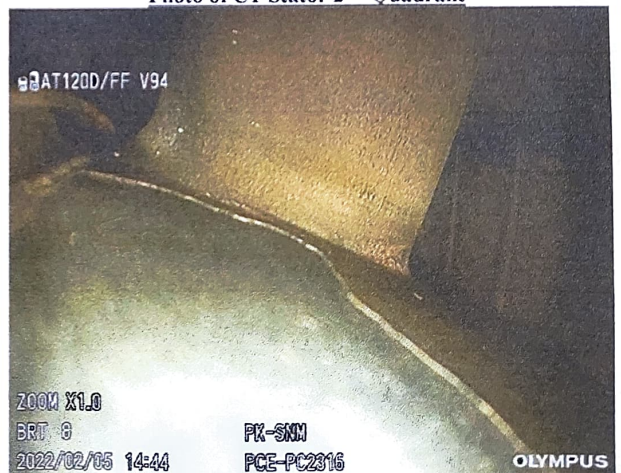
Photo of CT Stator 2 nd Quadrant
