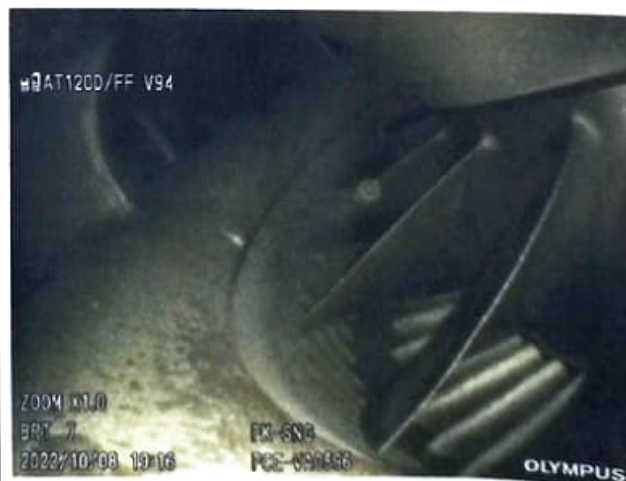
Photo of First Stage Compressor 2 nd Quadrant
