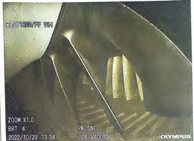
Photo of First Stage Compressor 4 th Quadrant
