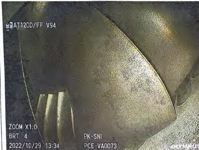
Photo of First Stage Compressor 3 rd Quadrant
