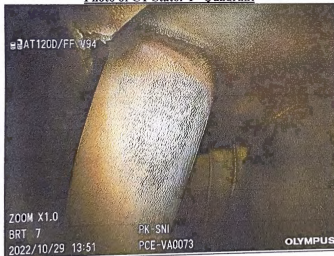
Photo of CT Stator 1 st Quadrant
