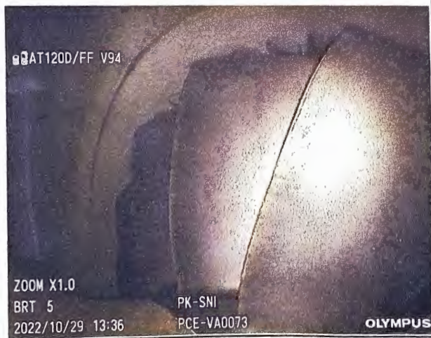
Photo of First Stage Compressor 1 st Quadrant
