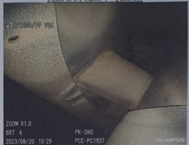
Photo of CT Stator 4 th Quadrant
