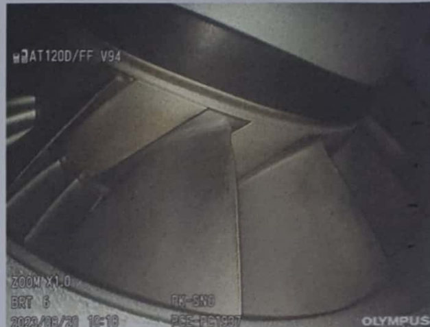
Photo of First Stage Compressor 4 th Quadrant
