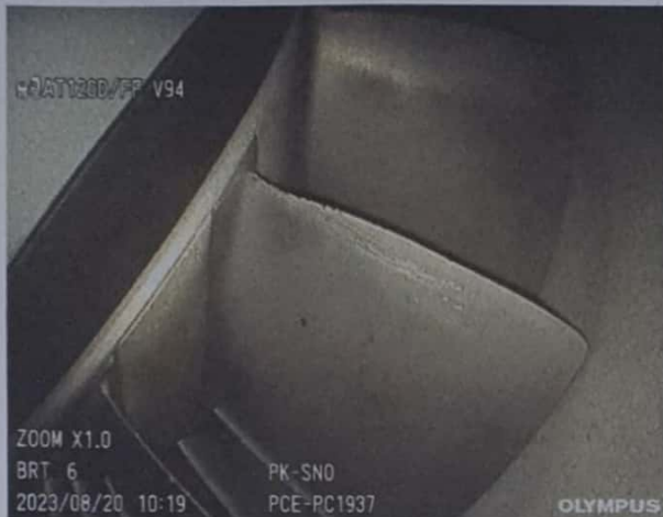
Photo of First Stage Compressor 3 rd Quadrant
