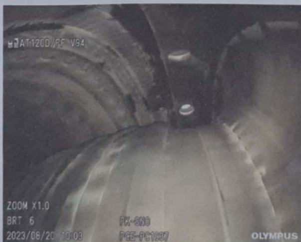
Photo of Combustion Chamber 1 st Quadrant
