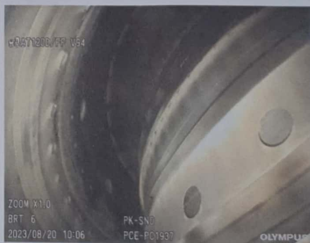
Photo of Combustion Chamber 2 nd Quadrant
