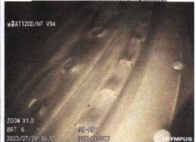
Photo of Combustion Chamber 2 nd Quadrant
