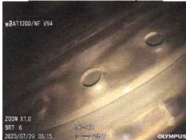
Photo of Combustion Chamber 1 st Quadrant
