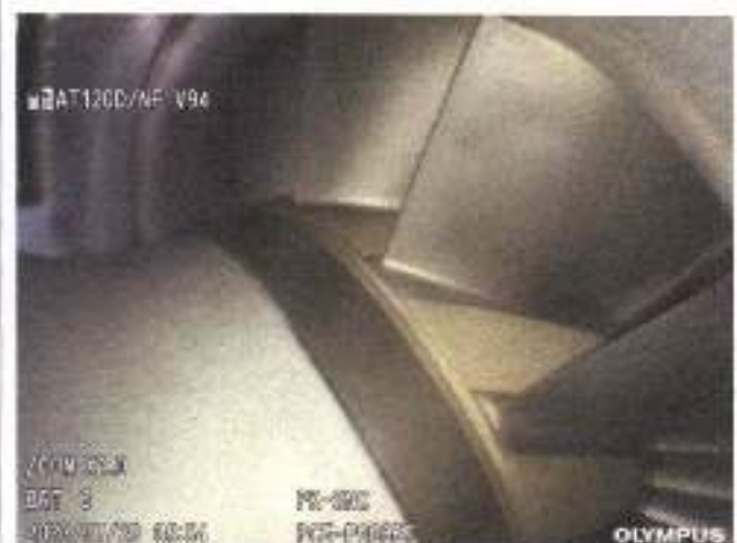
Photo of First Stage Compressor 2 nd Quadrant
