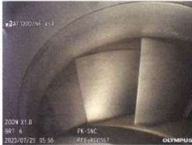
Photo of First Stage Compressor 3 rd Quadrant
