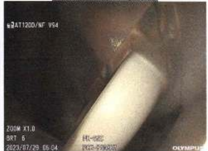
Photo of CT Stator 4 th Quadrant
