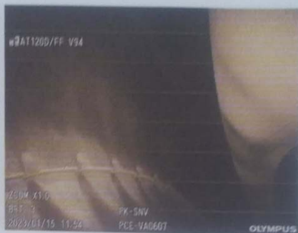
Photo of CT Stator 4 th Quadrant
