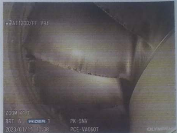
Photo of First Stage Compressor 4 th Quadrant
