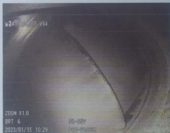
Photo of First Stage Compressor 1 st Quadrant
