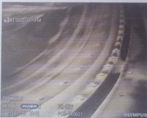
Photo of Combustion Chamber 1 st Quadrant
