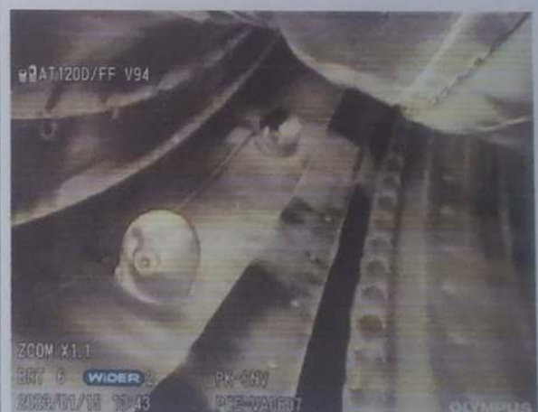
Photo of Combustion Chamber 2 nd Quadrant
