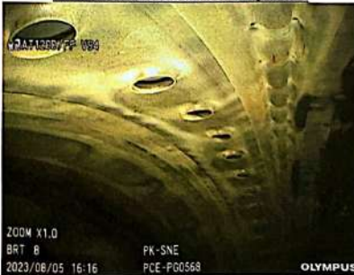
Photo of Combustion Chamber 2 nd Quadrant
