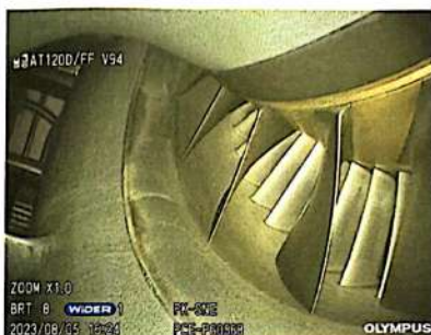
Photo of First Stage Compressor 4 th Quadrant
