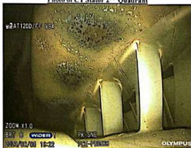
Photo of CT Stator 2 nd Quadrant
