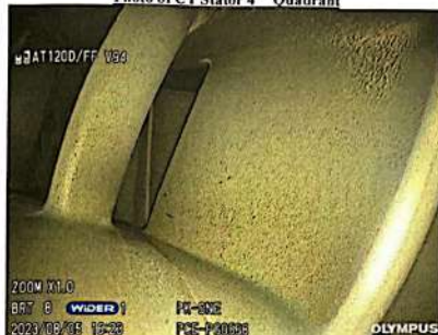
Photo of CT Stator 4 th Quadrant
