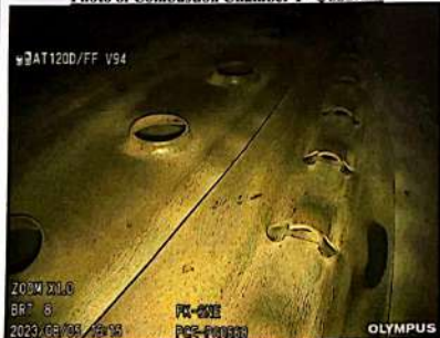
Photo of Combustion Chamber 1 st Quadrant
