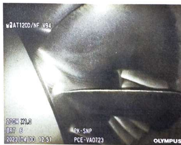
Photo of First Stage Compressor 2 nd Quadrant
