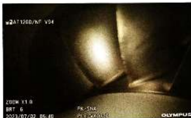
Photo of First Stage Compressor 4 th Quadrant
