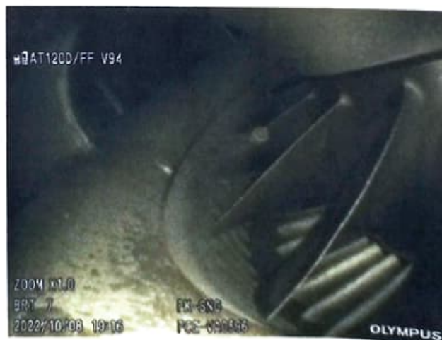
Photo of First Stage Compressor 2 nd Quadrant
