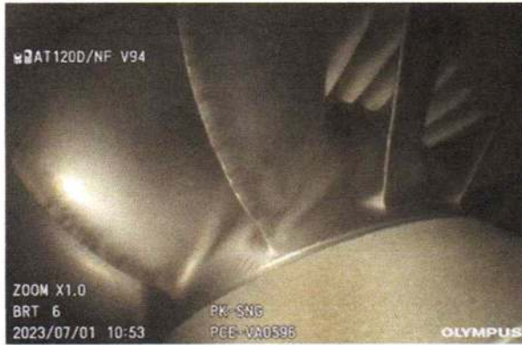
Photo of First Stage Compressor 3 rd Quadrant
