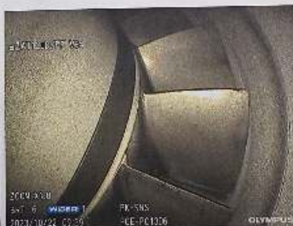
Photo of First Stage Compressor 1 st Quadrant
