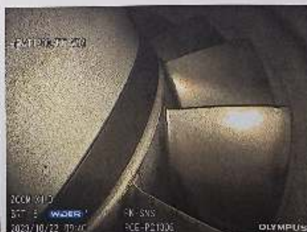
Photo of First Stage Compressor 2 nd Quadrant
